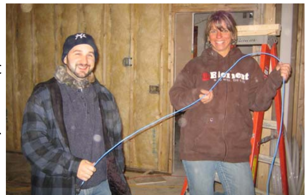
Pictured to the right: Brendon McGahan (Human Resources) and Vicki Kaan (IT Coordinator) work to install cable in early December.
